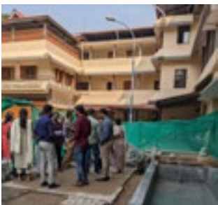
Mounting for nature inspired wastewater treatment at the Government Higher Secondary School in Kochi
