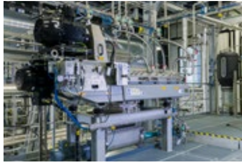
Decanter for separating suspended particles
