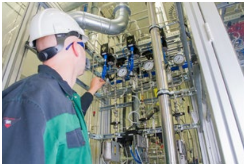
Upstream rack of the pilot plant for synthesizing methanol from synthesis gas
